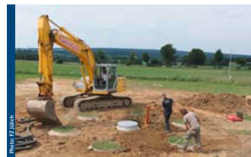
Six additional lysimeters are set up in a circle around every central measurement- and service shaft (top) Once the lysimeters have been set in place and the technology has been installed, the surrounding pit is filled in with soil (bottom)
